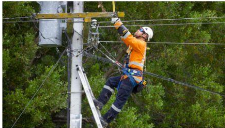
Unison faultman Dan Johansen working on power lines near Rissington. Photo / Warren Buckland
