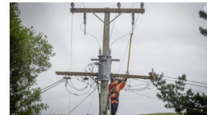
A Unison faultman working on power lines in Hawke's Bay following the cyclone. Photo / Warren Buckland
