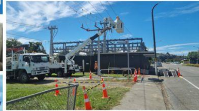
Electrical crews working to repair broken or damaged lines at the Taradale Rd switching yard. Photo / Lauren Crimp, RNZ
