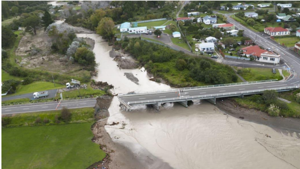
A section of the bridge in Tokomaru Bay has been wiped out by flood water, bisecting the town alongside State Highway 35 Photo: RNZ / Angus Dreaver
