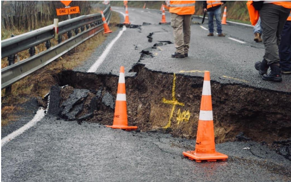
Slip site at Otoko, northwest of Gisborne. Photo: Kate Green / RNZ
