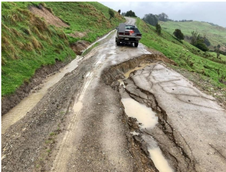
Waitangi Rd, Tairāwhiti, damaged in heavy rain. Photo / Supplied
