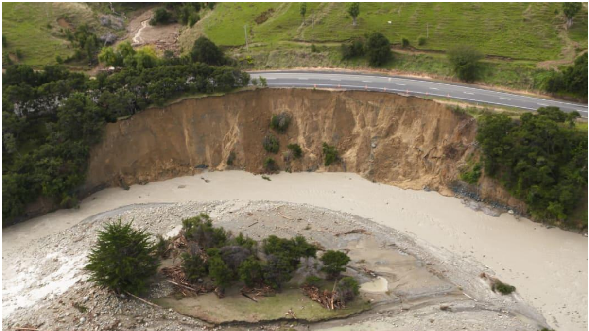
Mangahauini River eats away at State Highway 35 near Tokomaru Bay Photo: RNZ / Angus Dreaver
