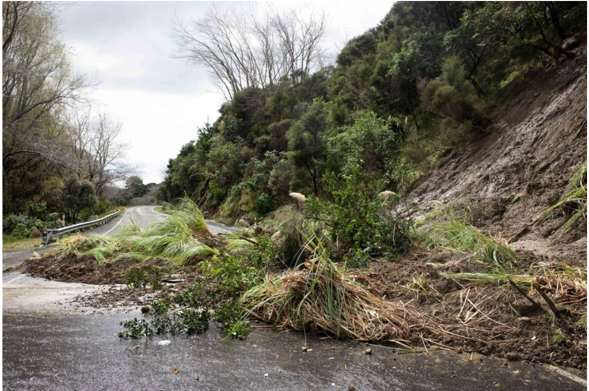
Slips cover the road along State Highway 35 Photo: RNZ / Angus Dreaver
