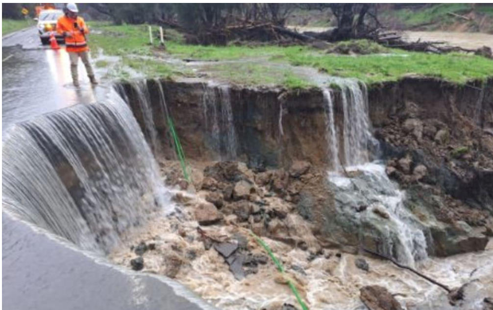
Heavy rain caused a slip on State Highway 35 north of Tologa Bay Photo: Supplied / Dion Milner
