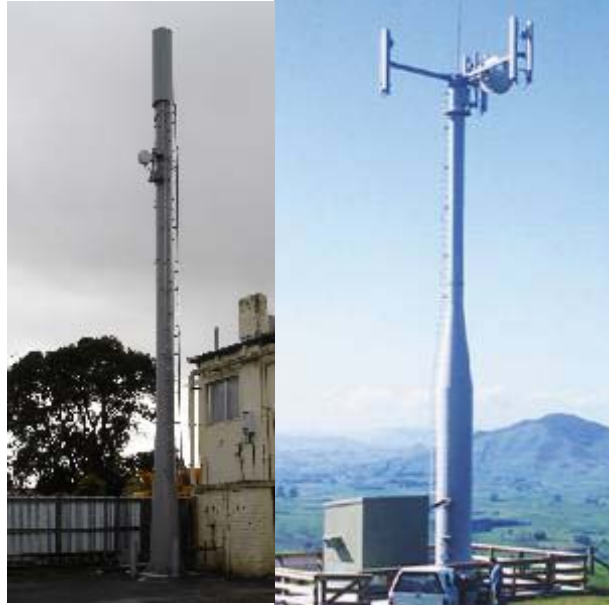
Figure 13.2 Typical masts for mobile services in New Zealand.
