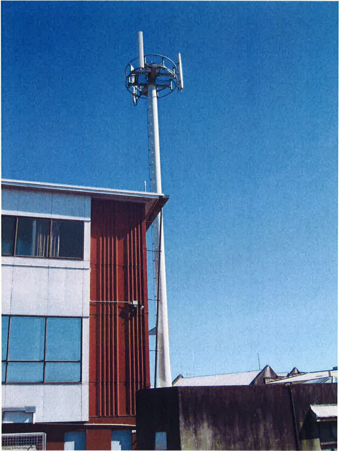
TNZ Te Awamutu Room for more antennas! Co-Lo request rejected due to structural reasons.
