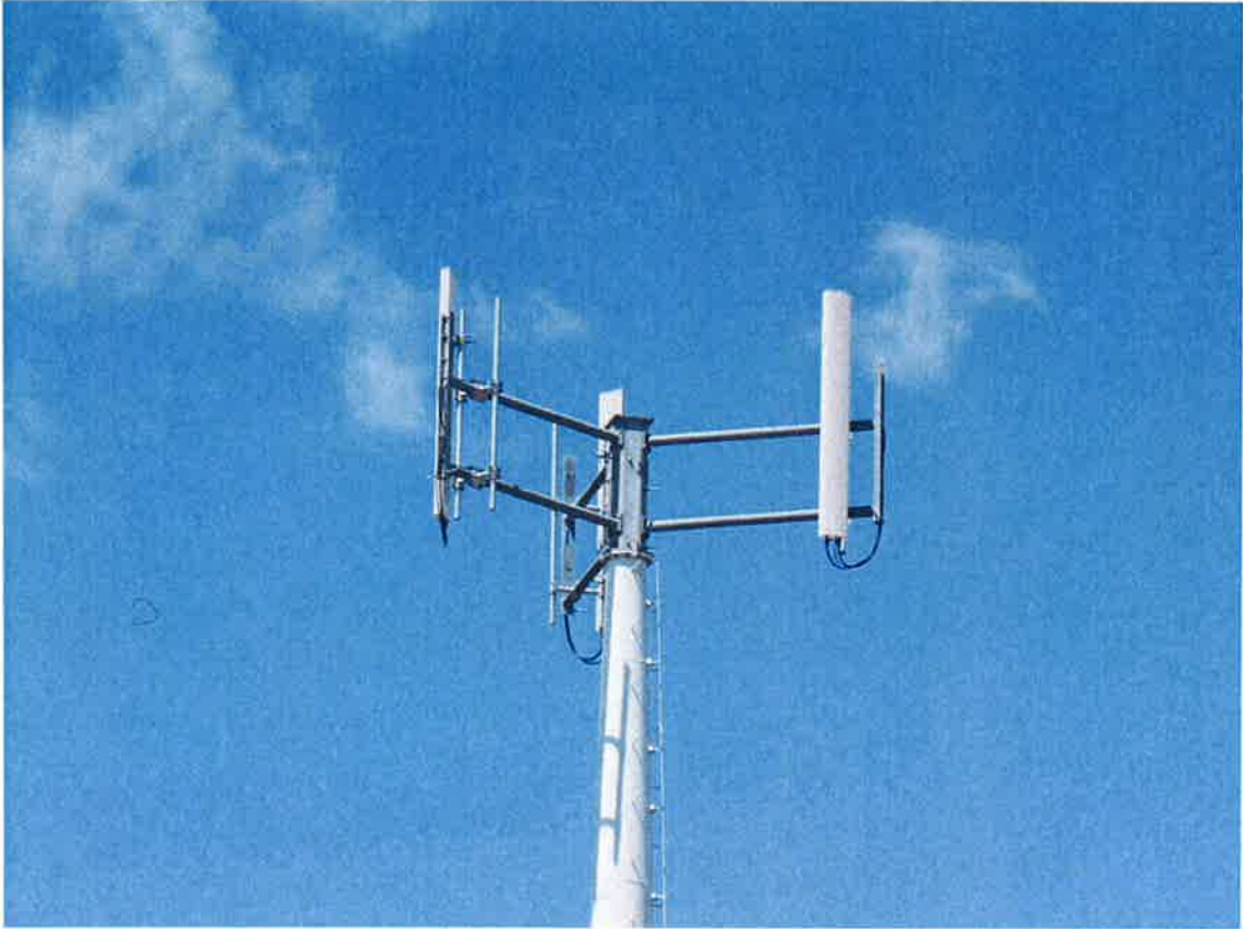
TNZ Matamata Exchange Close Up. 1 x-pol antenna per sector.
