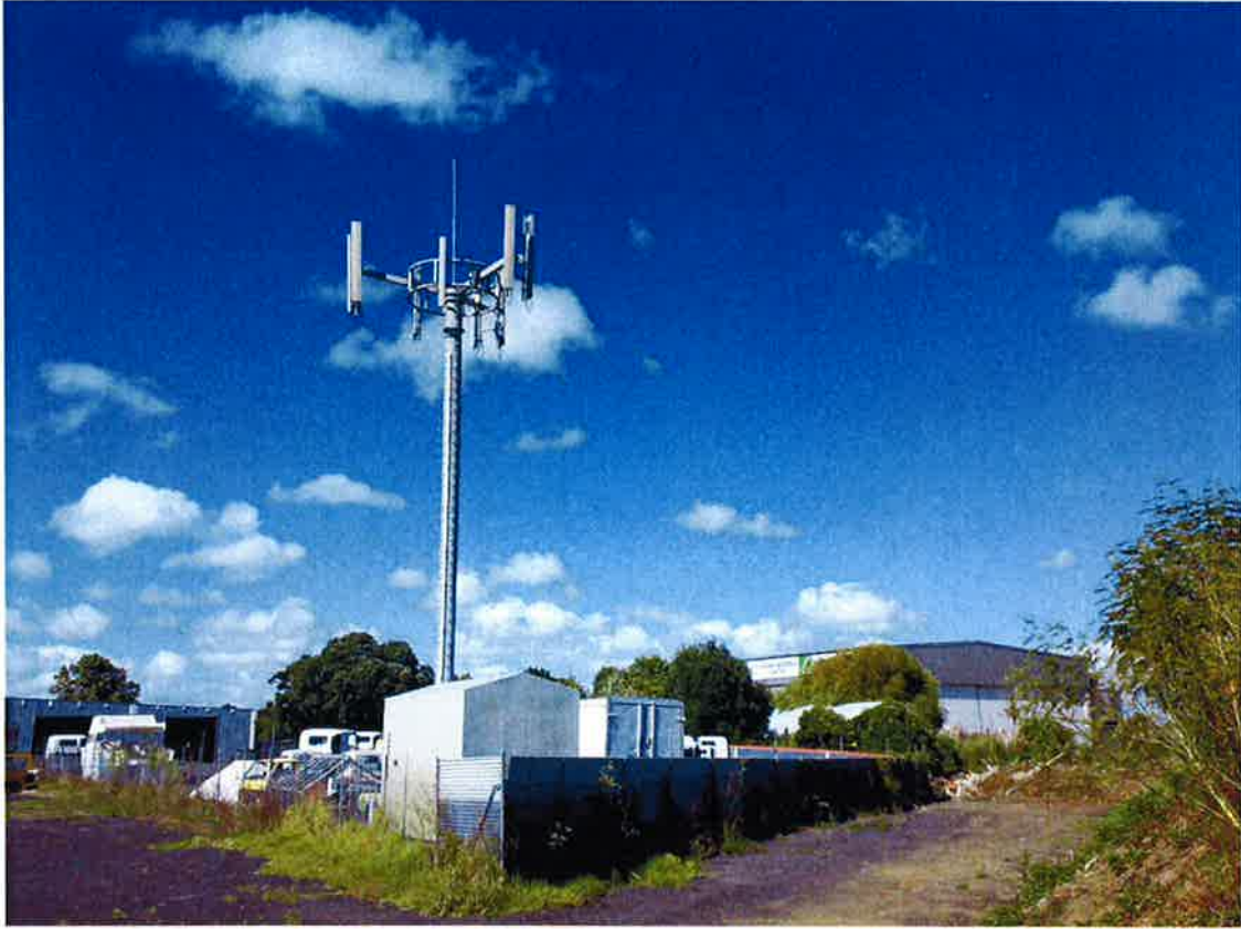
VNZ Otahuhu. Example of VNZ overlaying 3G services on an existing 2G site. 3G x-pol antenna (smaller) in centre of 2 x vertical-polarised antennas for 2G. There is room for NZC if VNZ swapped out 2 x vertical-polarised 2G antennas for 1 x-pol antennas
